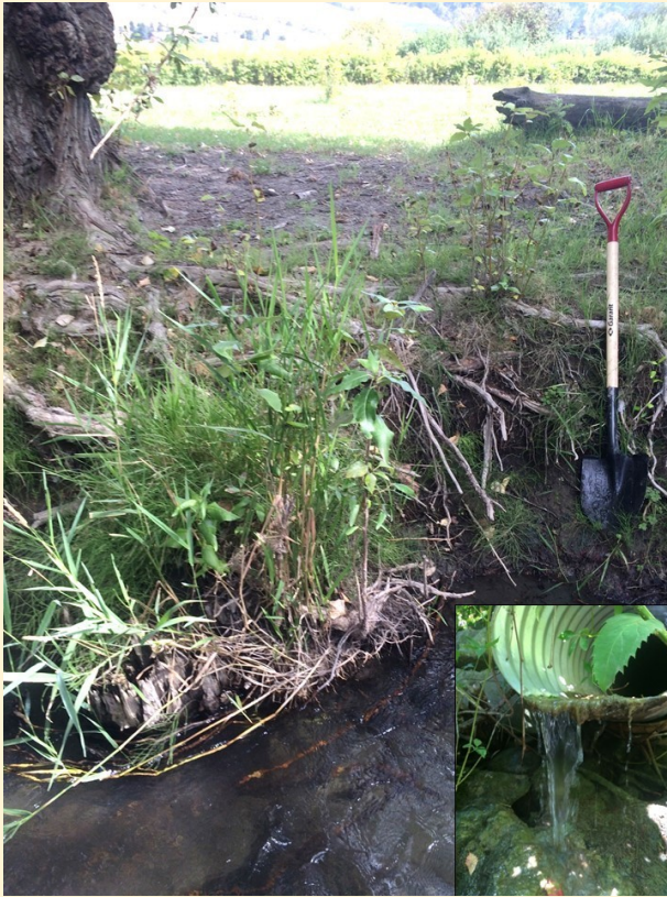
A degraded riparian area and a culvert along the creek.
