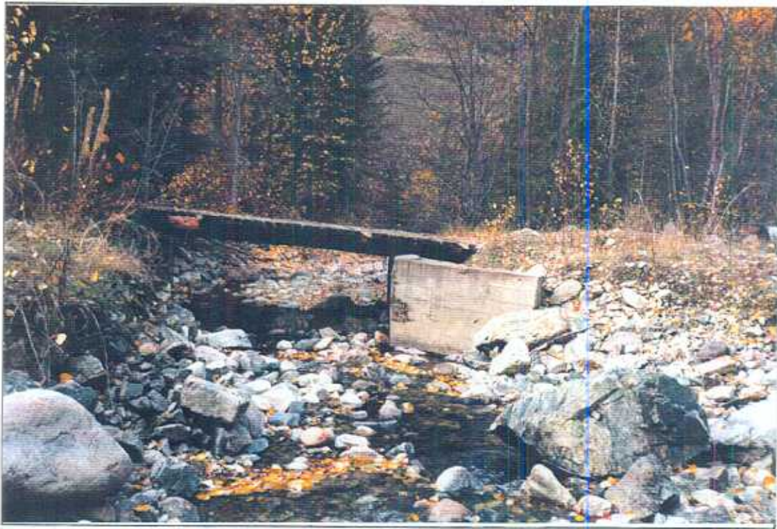
Photo 1. Bridge crossing at the rock quarry with some erosion around the abutments, downstream view.
