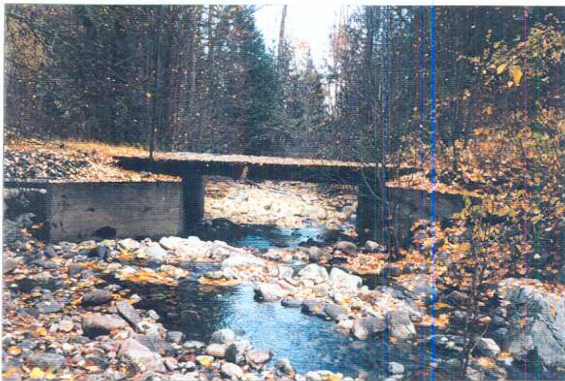
Photo 2. Bridge crossing 100m u/s from rock quarry with some erosion around the abutments, downstream view.
