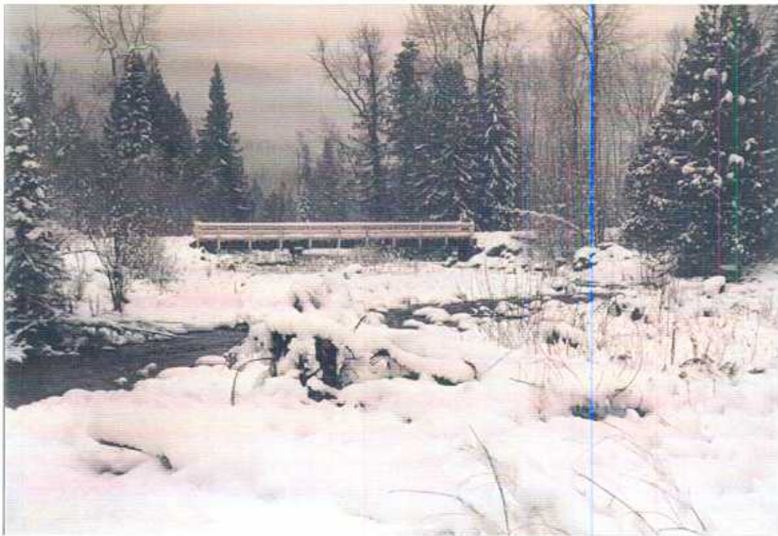
Photo 24. Bridge crossing with some LWD in the channel just u/s, downstream view. Stream Name: Mission Creek Site #: 51 Reach #: 7 GPS Coordinates: 49°53'25N 119°03'83W Code: Q•D•F•1
