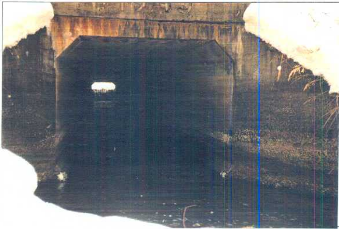
Photo 7. Concrete culvert (1.25m diam.) under the old railway bed of the KVR, upstream view. Stream Name: Hydraulic Creek Site #: 18 Reach #: 4 GPS Coordinates: 49°47'75N 119°12'04W Code: N/A
