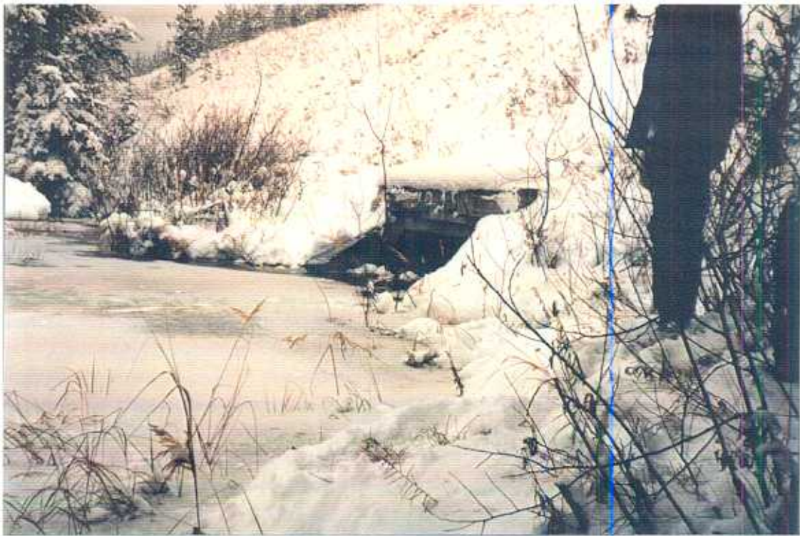
Photo 9. U/S end of the culvert showing 40cm opening remaining, downstream view. Stream Name: Hydraulic Creek Site #: 18 Reach #: 4 GPS Coordinates: 49°47'75N 119°12'04W Code: Fb•D•N•2
